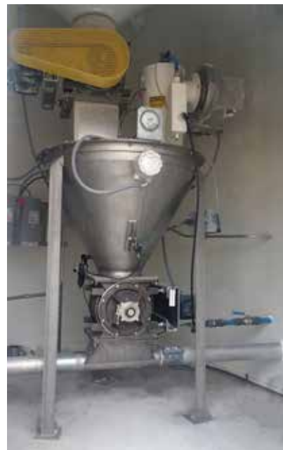
PNEUMATIC CONVEYING SYSTEM
